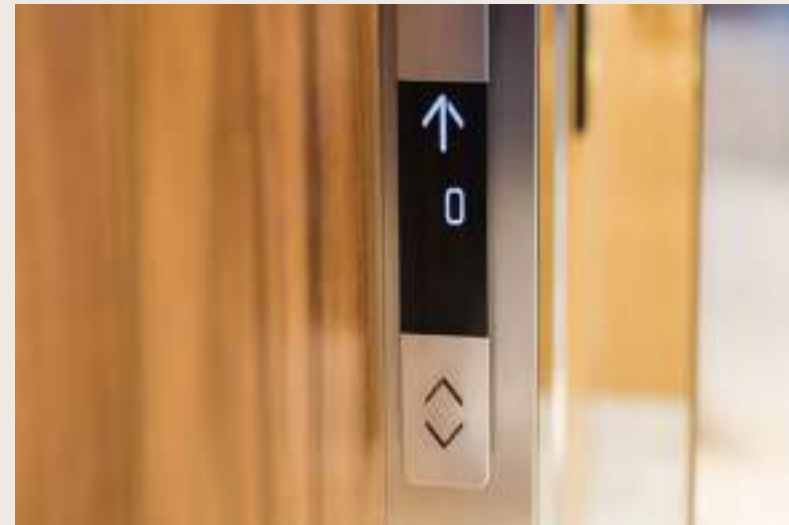
Elevator in each mansion
